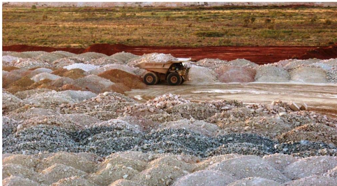
Figure 7-6: Paddock dumping MRS construction method, with darker coloured paddocks representing the fresher, sulfidic PAF rock, thereby also demonstrating encapsulation.
