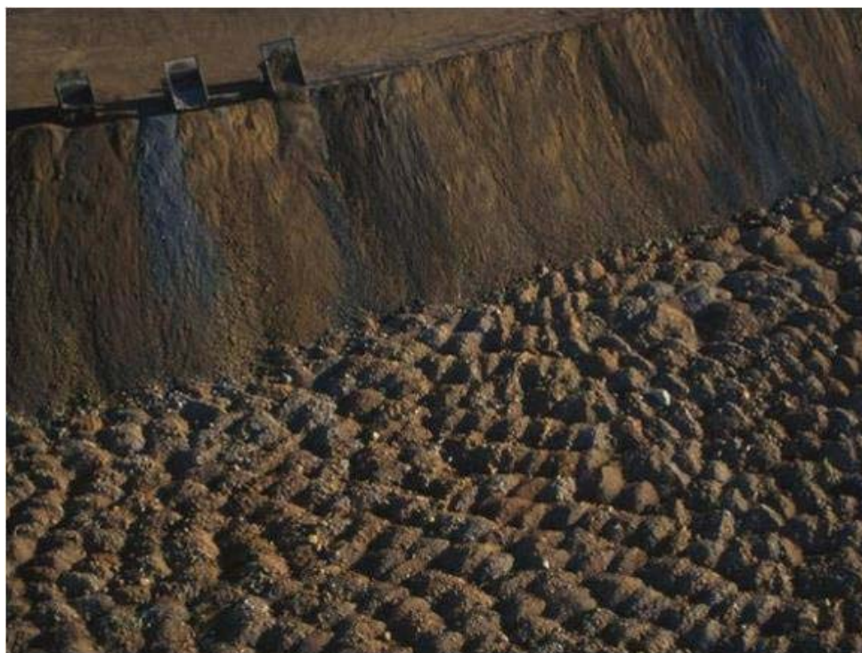
Figure 4-5: Combination of encapsulation and paddock dumping with base-up (thin lift) MRS construction methods. In this case, end-dumped PAF mine rock is being encapsulated by paddock-dumped NAF material. The paddock-dumped lifts are visible around the batters of the end-dumped PAF material in this image and will ultimately extend above the full height of the end-dumped material.
